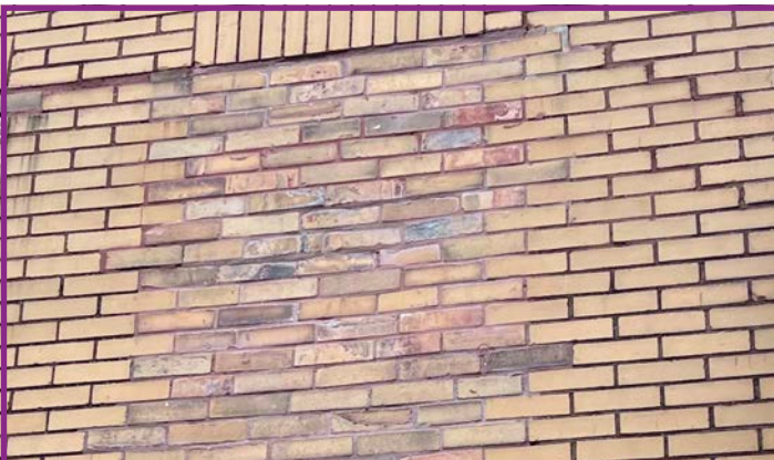
Window Opening Filled with Mismatching Brick (Color, Finish, Texture) and Mortar
