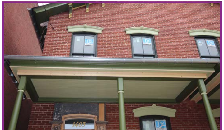
Structural Elements. The Porch Roof Rests on a Beam, and the Beam is Supported by Columns
