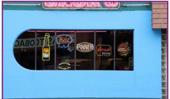
Altered Storefront Window that has Inappropriate Style and Form for a Historic District
