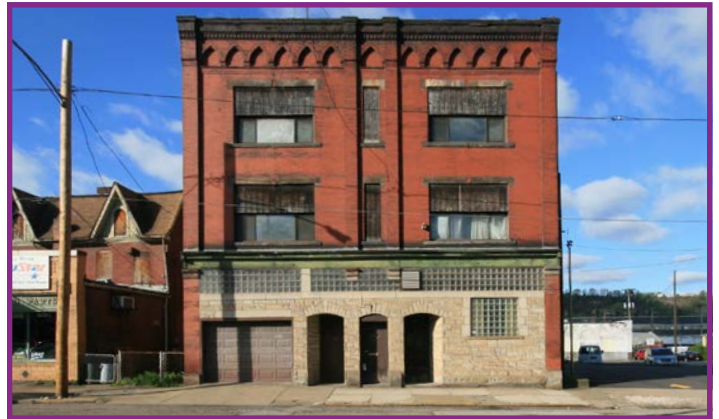
A Building with Unique Architectural Character that is in Need of Stabilization
