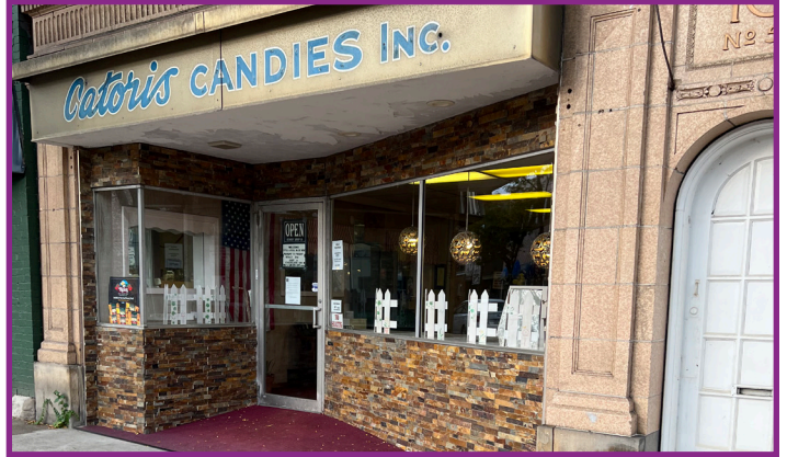
Historic Stone Commercial Building with New Inappropriate Stone Clad Storefront Infill (Bulkhead/Knee Wall)
