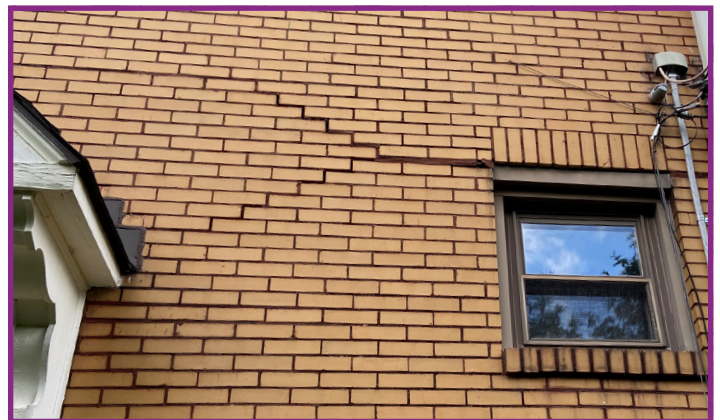
Rusted Steel Lintel Causing Masonry Damage and Water Infiltration into the Building's Structure
