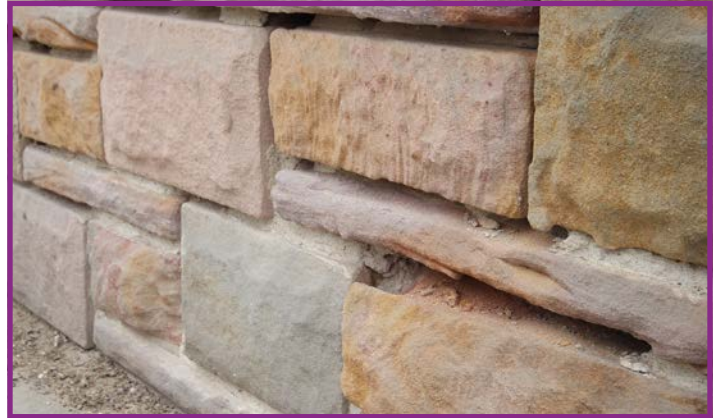
Washed Out Mortar Requiring Re-pointing to Preserve Long-Term Structural Integrity
