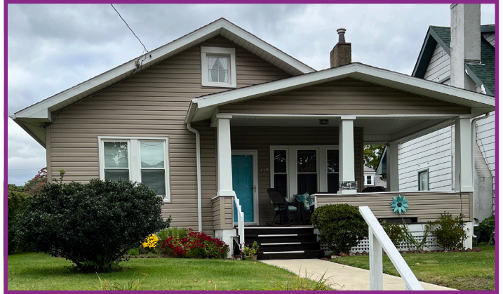
Vinyl Siding on a Historic Home Lacks the Character of the Original, Especially in the Trim Around the Windows and in Other Areas
