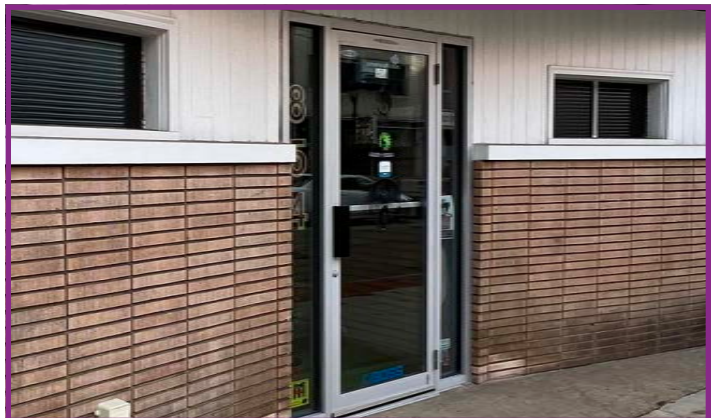
New Inappropriate Storefront Door for Historic Commercial Building
