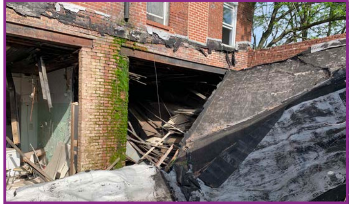
Deteriorated Structure that Poses a Danger to Life
