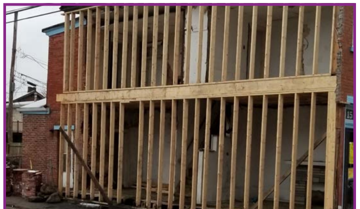
Structural Elements. New Two-Story Frame Wall, Studs (Vertical) and Band Joist (Horizontal)
