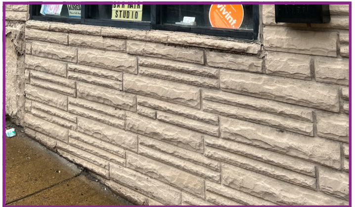
Storefront Clad in Inappropriate Stone Veneer
