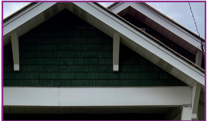
Aluminum Wrap Covering Existing Wood Trim was Heavily Marketed for Decades, but has Significantly Less Detail than the Original
