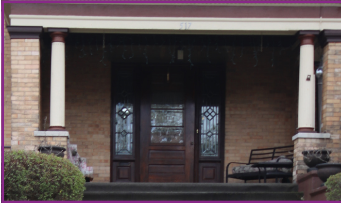
Historic Wooden Door with 2/3 Glass and Sidelights on Both Sides of the Door
