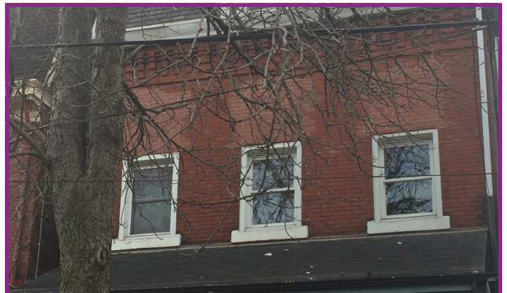
Original Window Openings have been Partially Filled with Brick to Alter the Windows' Size
