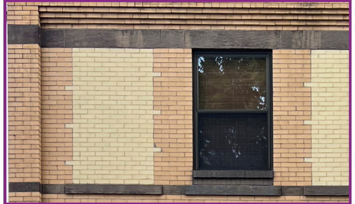
Infilled Window with Mismatching Brick
