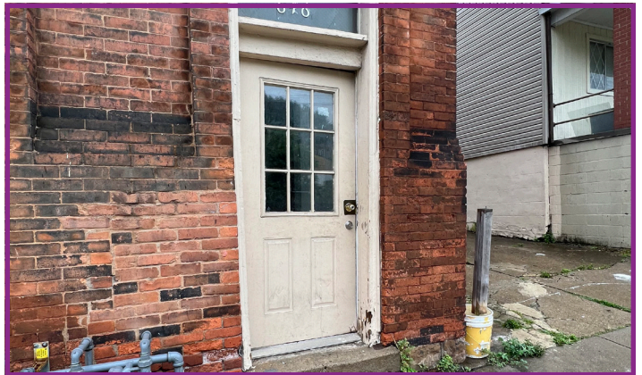
Original Door Opening Filled with Standard, Inappropriate Style Door
