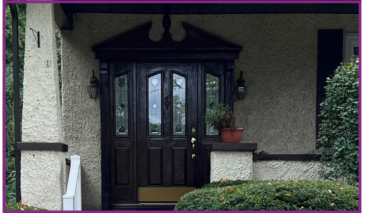
Inappropriate New Entry Door, Not Historically Accurate Style and Inappropriate for the House's Architectural Style
